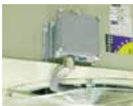
Outside connecting box.
